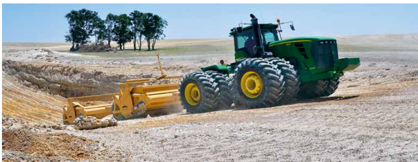
Spreading is more cost-effective when the clay pit is close to the area to be treated.
